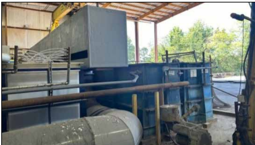
TUBE & PIPE HOT DIP PICKLING LINE
