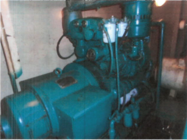
Starboard side generator
