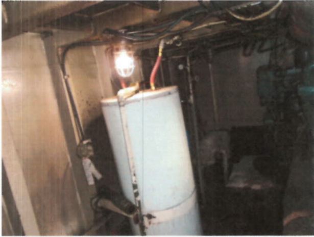
Water heater on the port side of the machinery space
