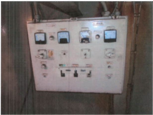
Main generator panel on the forward bulkhead in the machinery space
