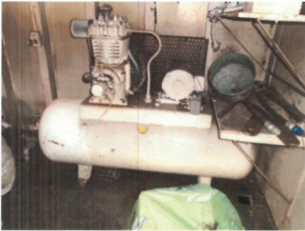
Aft air compressor
