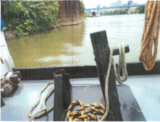
Damaged "H" Bit
