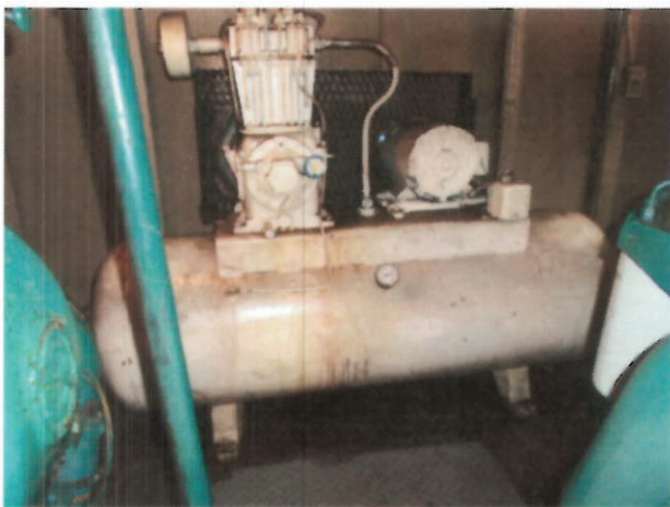
Forward air compressor
